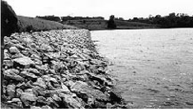
Figure 3. Rock riprap may be required to protect a dam from wave action, especially if the dam faces the prevailing wind or has a large pond.
