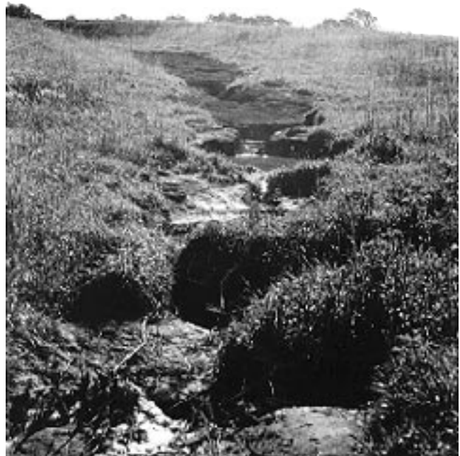
Figure 9. A livestock path can cause failure of the grass cover in the emergency spillway and, ultimately, if not repaired, dam failure.
