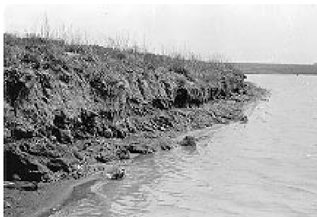
Figure 1. Wave action can cause excessive erosion to the face of the dam.
