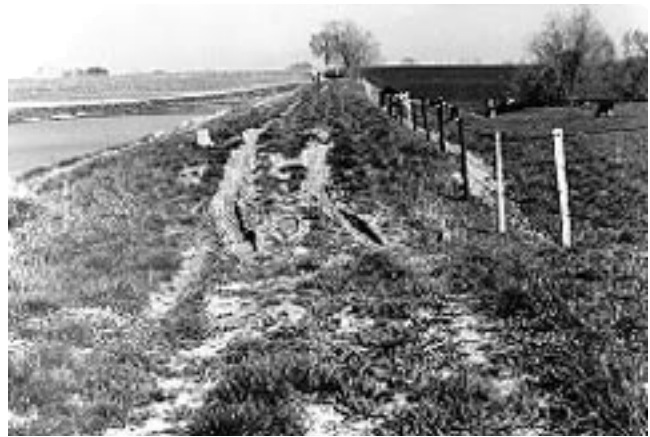
Figure 8. Keep livestock fenced away from the dam and the emergency spillway to maintain a vigorous vegetative cover for erosion control.
