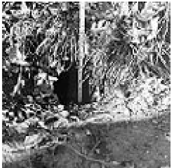
Figure 6. Eliminate animal burrows in the dam to prevent failure.
